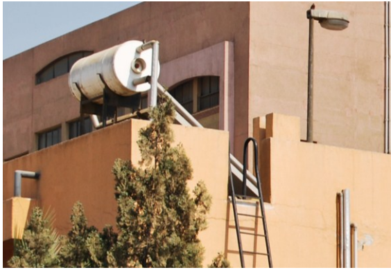
An Egyptian SWH in operation
