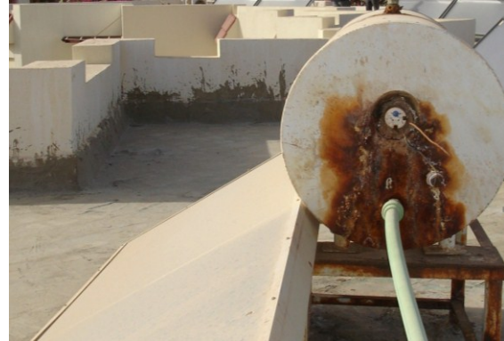
Corrosion of solar water heater tank
